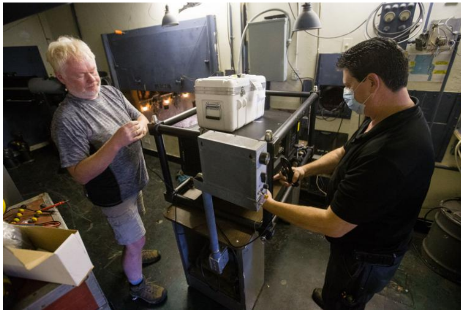
Craig Hoerig, left, and Gary Cooper install a new projector at the Keith-Albee Performing Arts Center on Tuesday, Aug. 18, 2020, in downtown Huntington.
